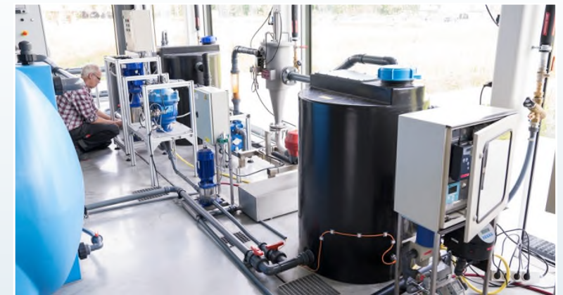
SCREENS FOR RO PRETREATMENT
