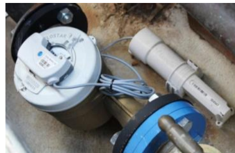
Smart customer meter
