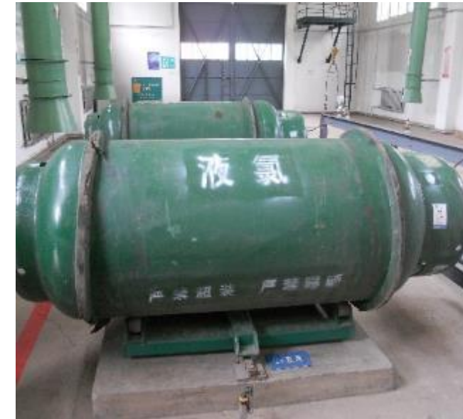
Liquid chlorine tank
