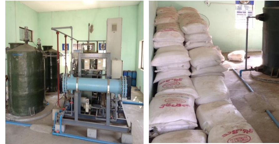
Electrolyzer (left) and Salt bags for chlorination process (right)
