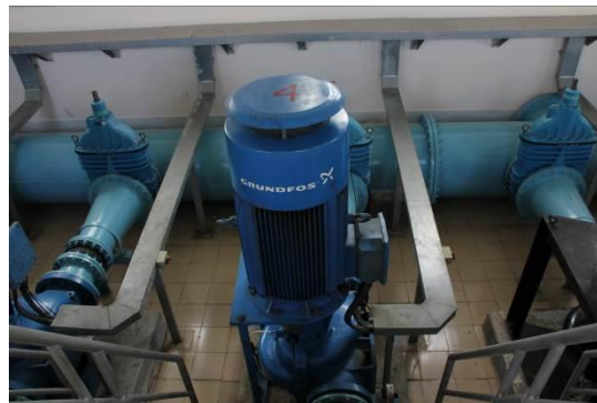
Distribution pump (black) and backwash pump (blue)
