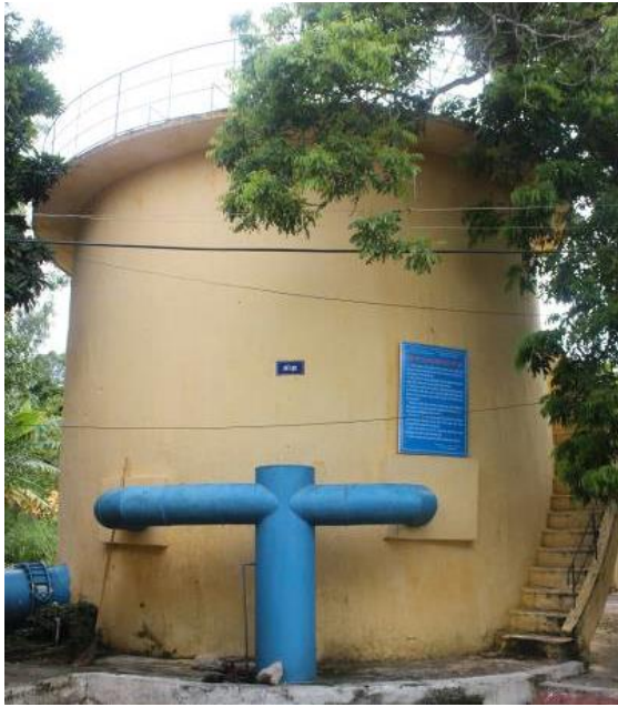
Circular filtration tank
