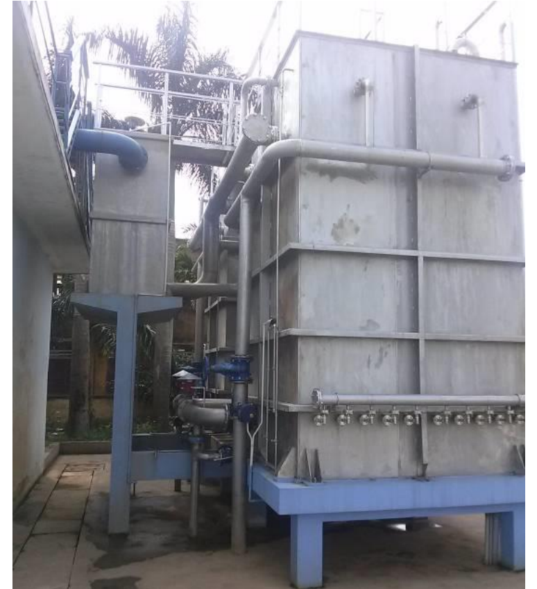
Biological Contact Filter
