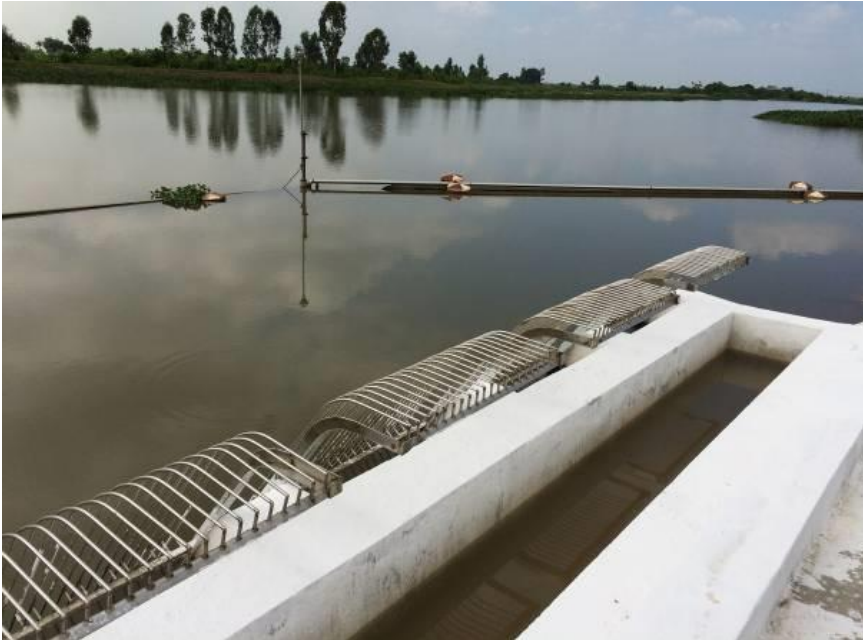
Raw water collection at Da Do river
