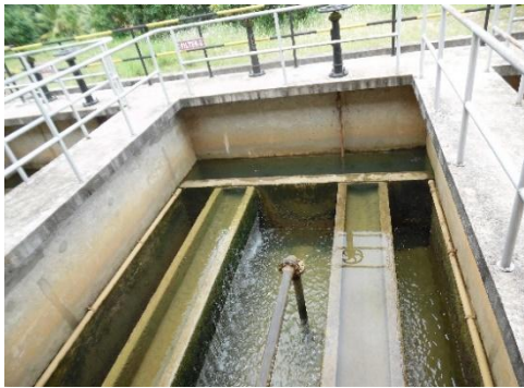
Figure 7a Filter (4 units)
