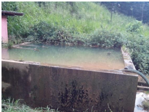
Figure 8a Sludge thickener
