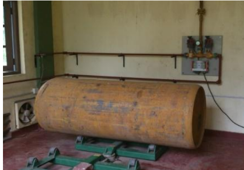
Figure 3 Gas chlorine cylinders (900 kg)
