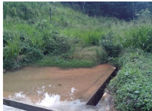
Figure 8b Sludge drying beds (3 units)
