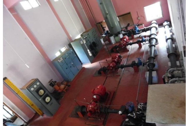
Figure 9 Treated water pump house
