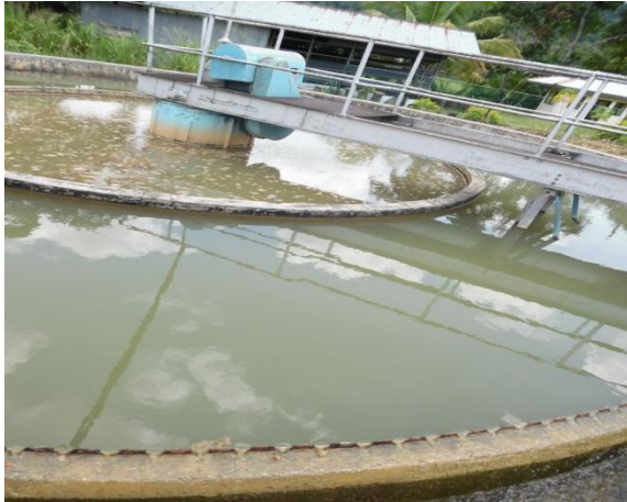
Figure 7a Clari-flocculator (2 units)
