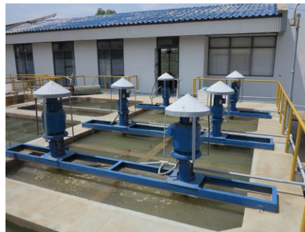
Figure 14 Mechanical flocculator (not operating)
