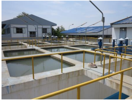
Figure 8 Sedimentation Tank (4 basins)
