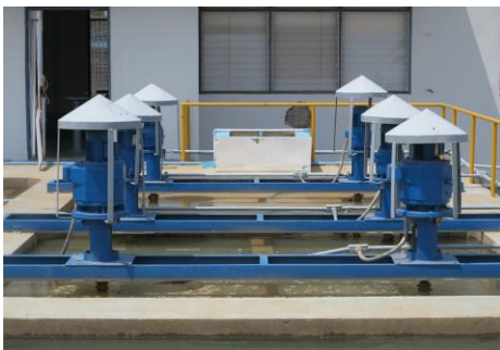
Figure 6 Mechanical Mixing (3 basins)
