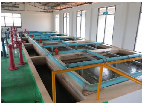
Figure 10 Filter Tank (7 basins)
