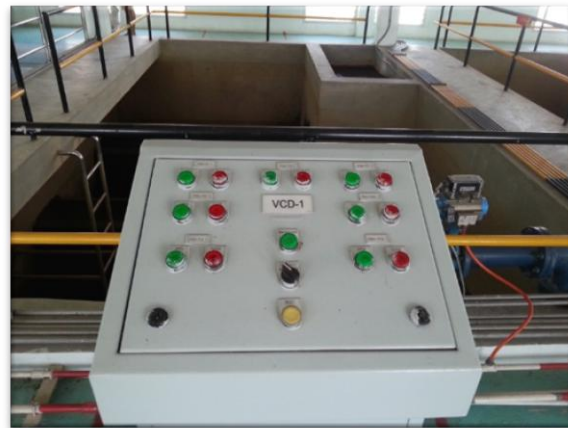
Figure 9 Filter Control Panel
