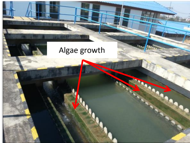
Figure 13 Sedimentation Basin with Algae Attached
