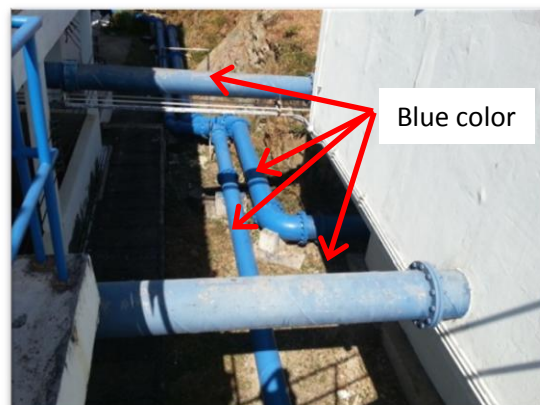
Figure 15 Pipeline Color of Nakhon Sawan WTP
