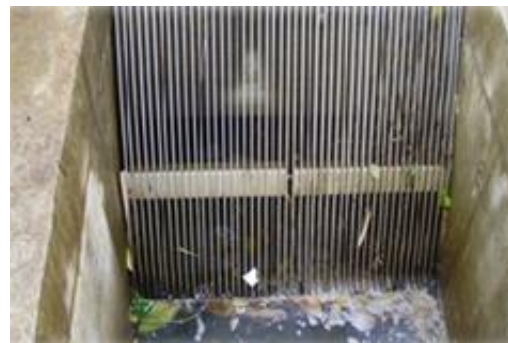
Figure 3 Screens of Intake
