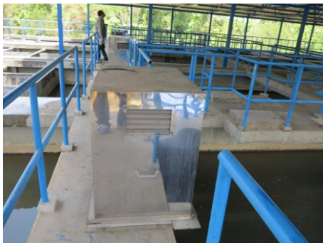
Figure 15 Mechanical Sludge Collector Motor
