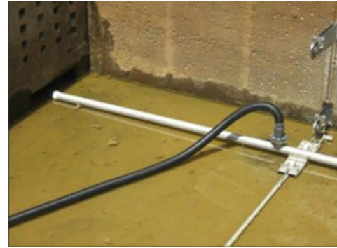
Figure 8 Sludge Collector System
