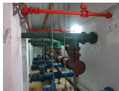
Figure 19 Identification of Pipe Line
