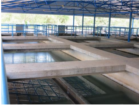
Figure 7 Sedimentation Tank (4 basins)
