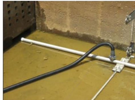
Figure 16 Sludge collector System (Leopold CT2 type)
