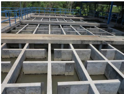
Figure 5 Flocculation Tank (4 basins)
