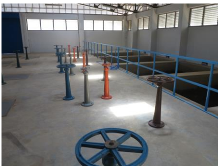
Figure 9 Filter Tank (10 basins)
