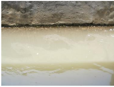
a) Flocculation basin
