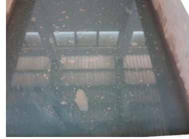
c) Surface water of filter basin
