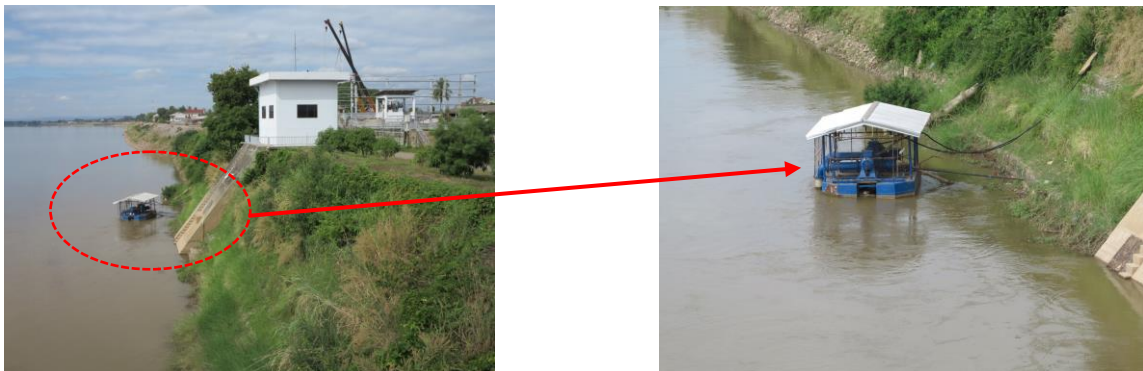
Figure 16 Floating Water Intake Pump
