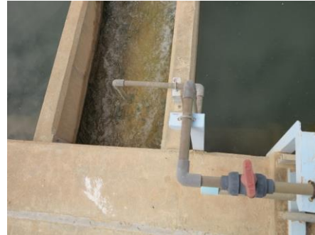
Figure 10 Injection Line of Pre-chlorination
