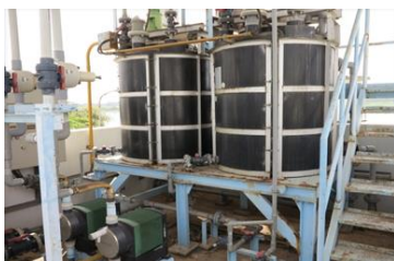
Figure 4 Polymer Storage Tank
