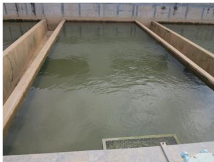
Figure 11 Filter Tank (8 basins)
