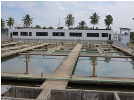
Figure 9 Sedimentation Tank (8 basins)
