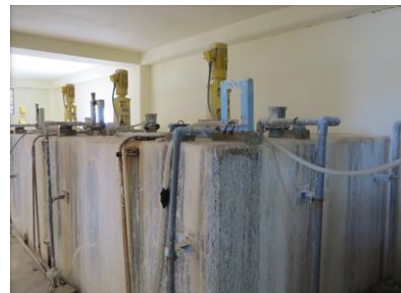
Figure 3 Chlorine Solution Tank
