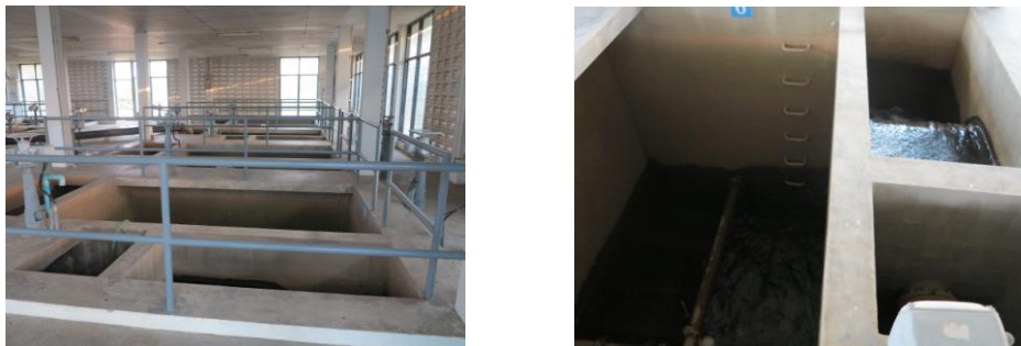
Figure 9 Filter Tank and Entrance Part of Filter
