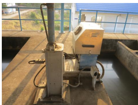
Figure 13 Mechanical Sludge Collector Motor
