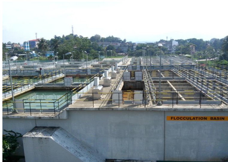
Figure 10 Side View of Flocculation Basin (160 chambers)
