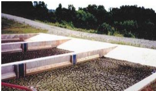
Figure 13 Sludge drying bed
