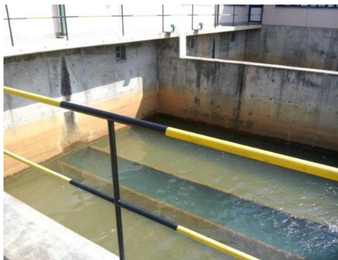
Figure 12 Rapid Sand Filter
