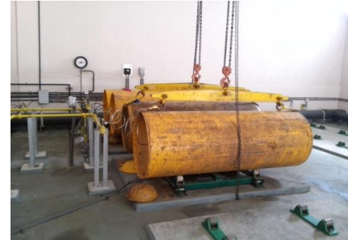
Figure 6 Gas Chlorine Cylinders (1700kg)
