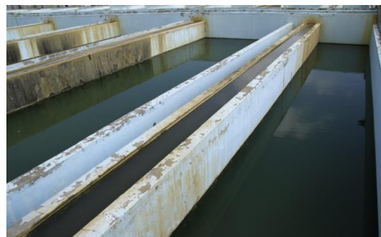
Figure 5 Sludge Blanket Sedimentation Tank
