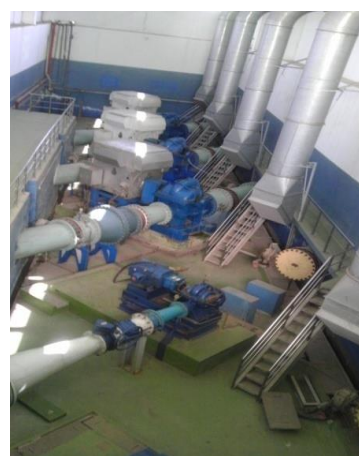
Figure 9 Clean water pumping station
