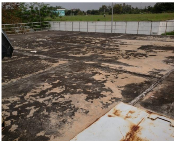
Figure 8 Clean water reservoir
