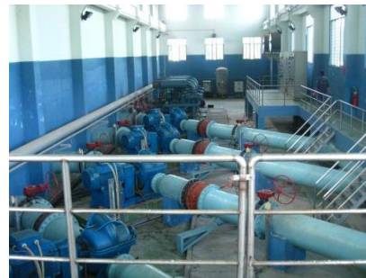
Figure 7 Air pump system for filtration tank
