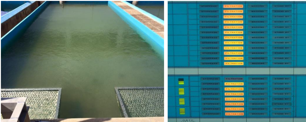
Figure 7 Filtration tank and control panel
