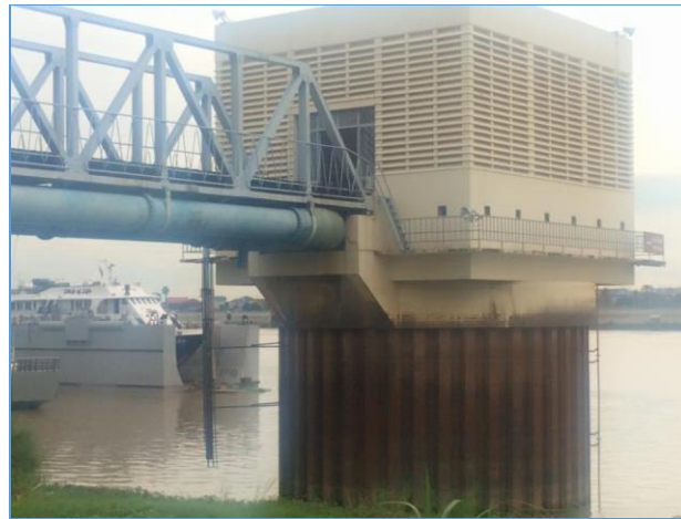
Figure 3 Raw water intake station
