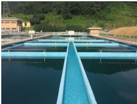
Figure 8 Sedimentation Tank (12 basins)
