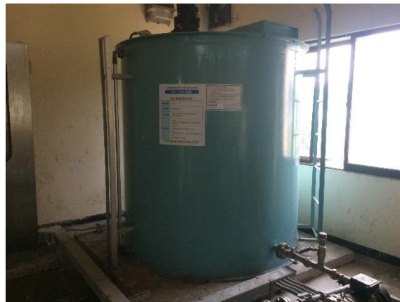
Figure 5 Polymer Storage Tank for Dewatering Aid (emulsion)
