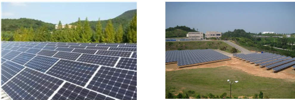
Figure 16 Solar Panels Installed in K-water
