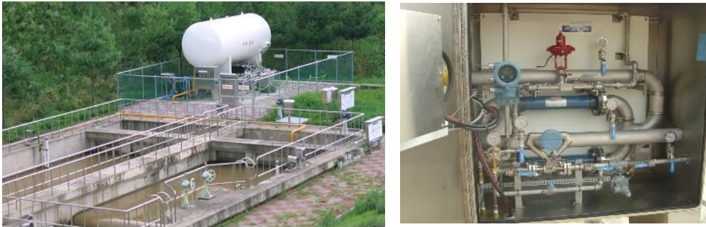
Figure 15 Facility of carbon dioxide injection in Dukso WTP
