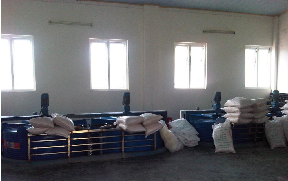
Figure 6 Chemical Mixing Tanks
