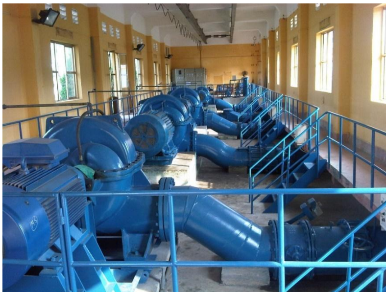
Figure 11 Pumping Station No. 1
