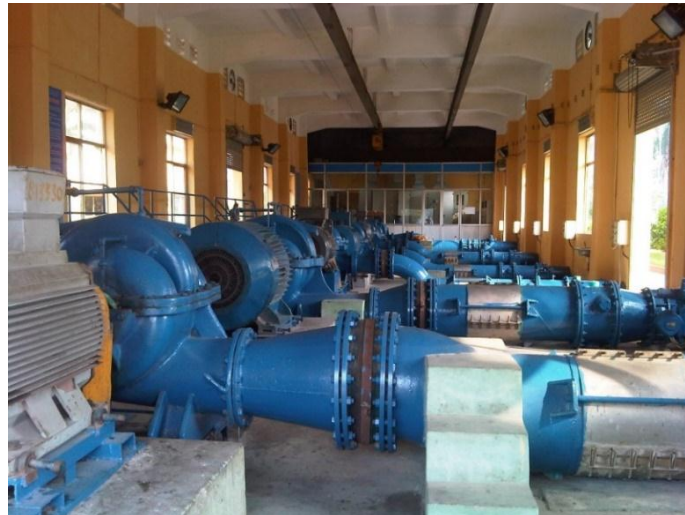
Figure 12 Pumping Station No. 2
