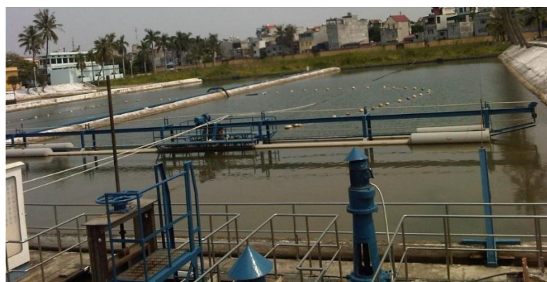
Figure 9 Horizontal Sedimentation Tank
