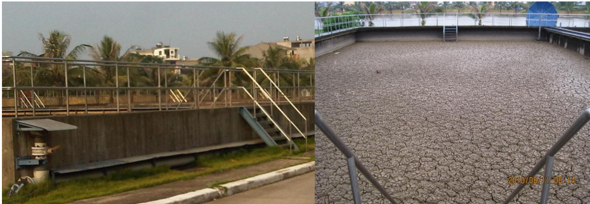
Figure 15 Sludge Drying Beds
