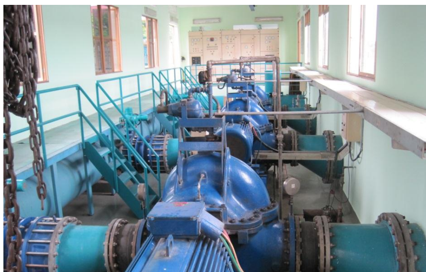
Figure 3 Quan Vinh Pumping Station
