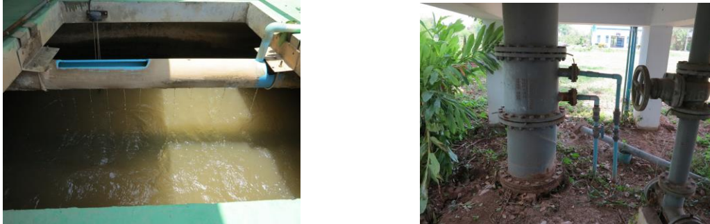
Figure 4 Hydraulic jump of alum (left) and static mixing of pre-chlorine (right)
