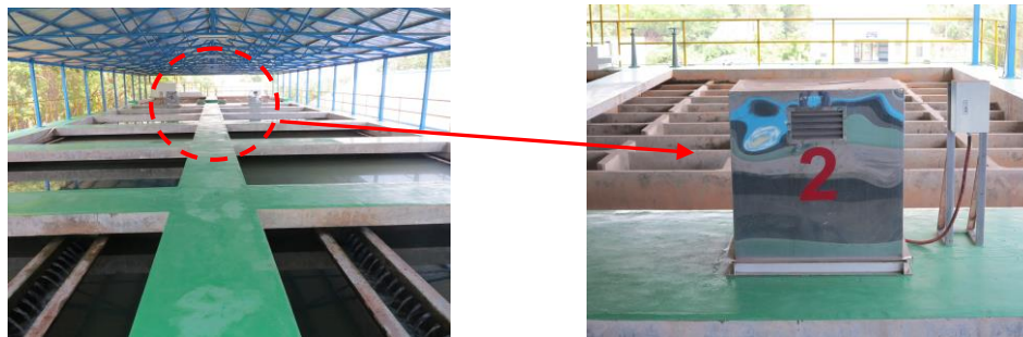
Figure 8 mechanical sludge collector (2 nd WTP sedimentation basin)
