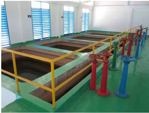
Figure 18 Manual operated valve (1 st WTP)
