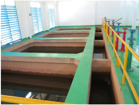
Figure 9 Filter Tank (10 basins)
