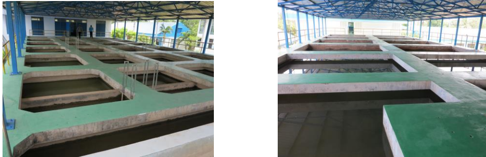
Figure 7 1 st WTP sedimentation basin (left) and 2 nd WTP sedimentation basin (right)
