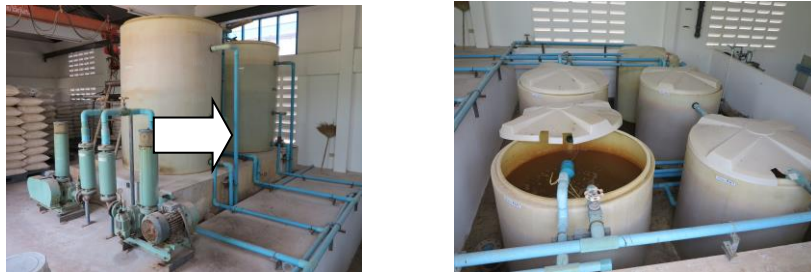
Figure 2 Alum Solution Tank (left) and storage tank (right)
