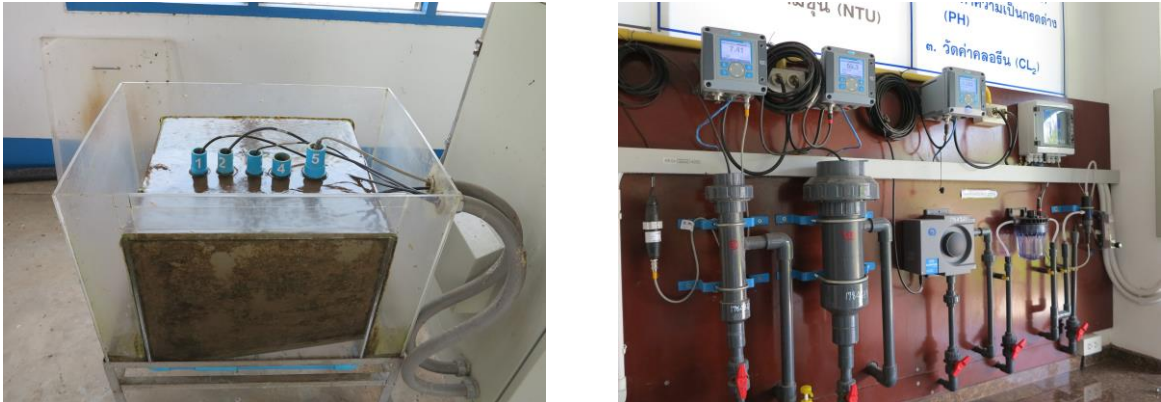
Figure 20 On-line monitoring devices: raw water (left) and treated water (right)
