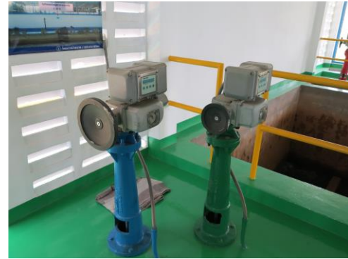
Figure 19 Motor-operated valve (2 nd WTP)
