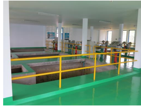
Figure 10 Elevated tank for backwashing (250 m 3 )
