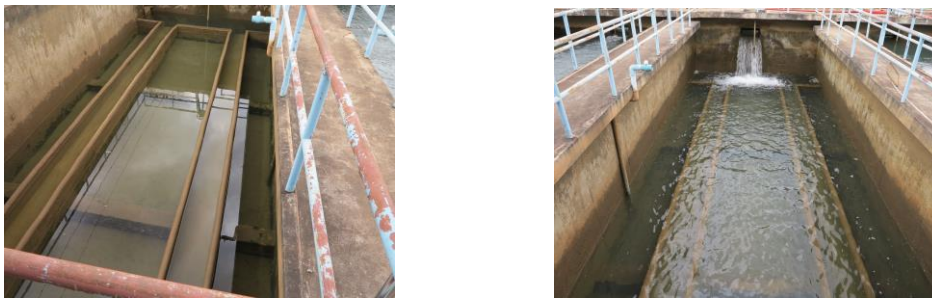
Figure 6 Filter Tank (5 basins)
