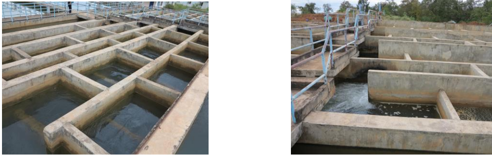
Figure 4 Vertical baffle channel (2 basins)
