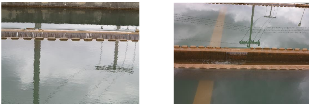
Figure 7 Damaged V notch weir
