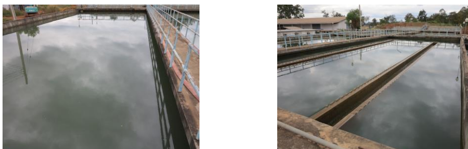
Figure 5 Settling part (left) and effluent part (right) of sedimentation tank (2 basins)
