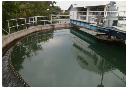
Figure 12 Sludge thickener (3 basins)
