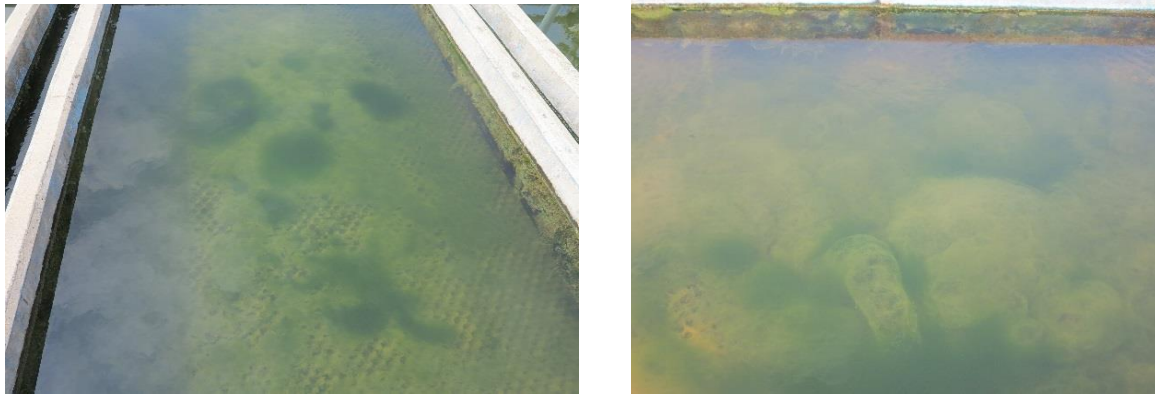
Figure 17 Excessive algae growth in clarifier basins
