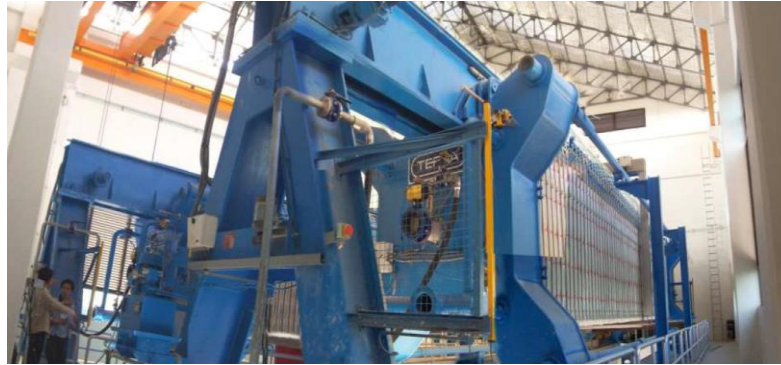
Figure 13 Filter press (2 units)
