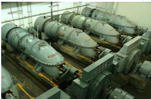
Figure 2 Samlao raw water pumping station
