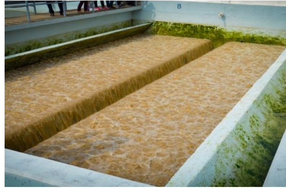
Figure 8 Backwashing with air scouring
