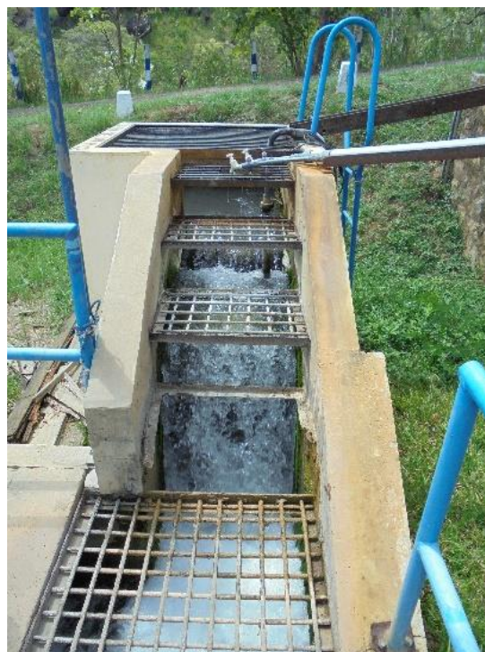
Figure- 3: Chemical adding point
