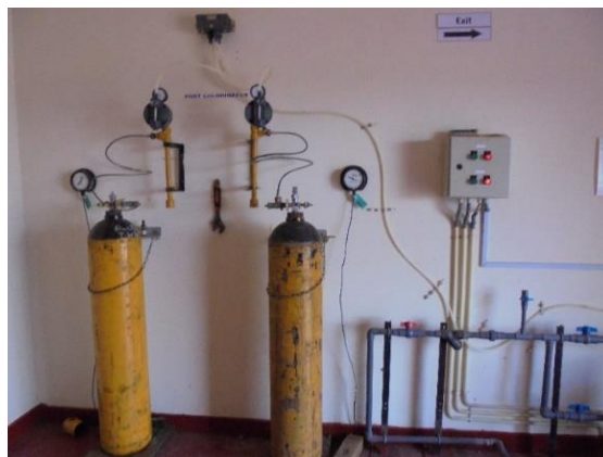
Figure-7: Gas chlorine adding system
