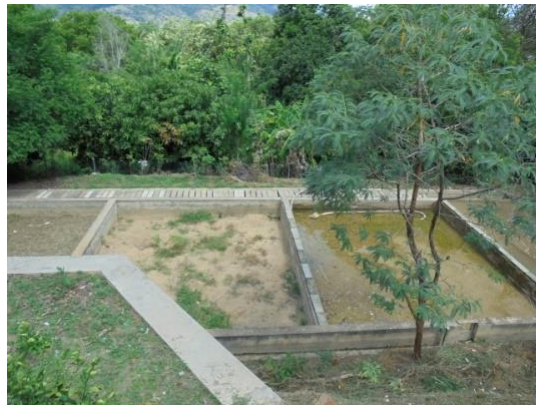
Figure-8: Sludge drying beds
