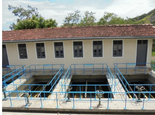
Figure -6: Filtration units
