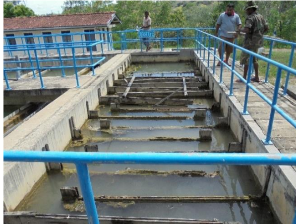
Figure-4 Flocculation tank
