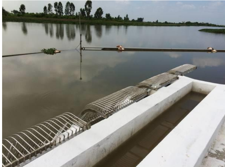
Figure 2 Raw water collection at Da Do river
