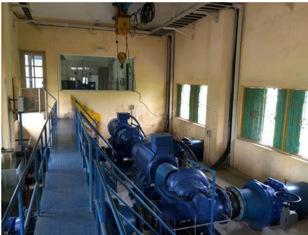
Figure 8 The second pumping station
