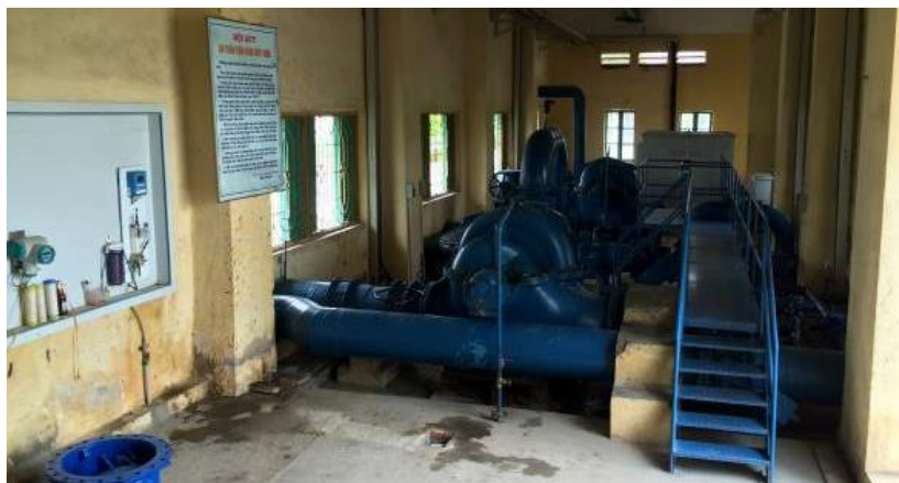
Figure 7 Pumps used in the first pumping station and backwash pumping station
