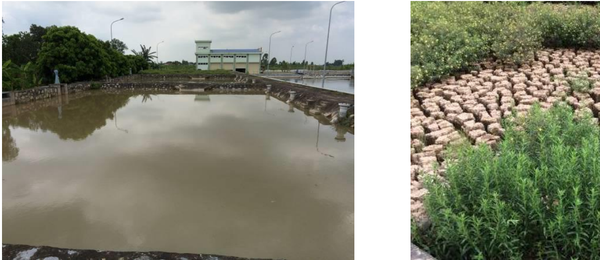
Figure 11 Sludge drying bed
