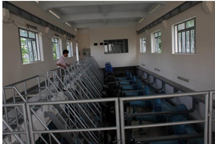
Figure 10 Secondary pumping station
