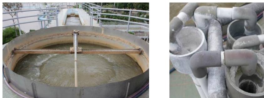
Figure 2 Chemical mixing tank and Lime & PAC adding facility
