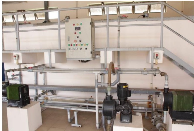
Figure 15 Chemical dosing pump
