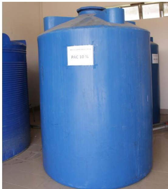
Figure 14 PAC storage tank
