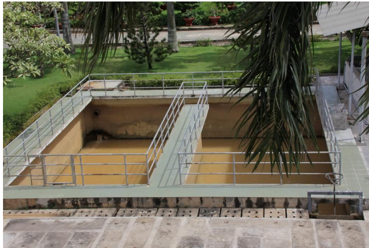
Figure 13 Backwashed water collection tank
