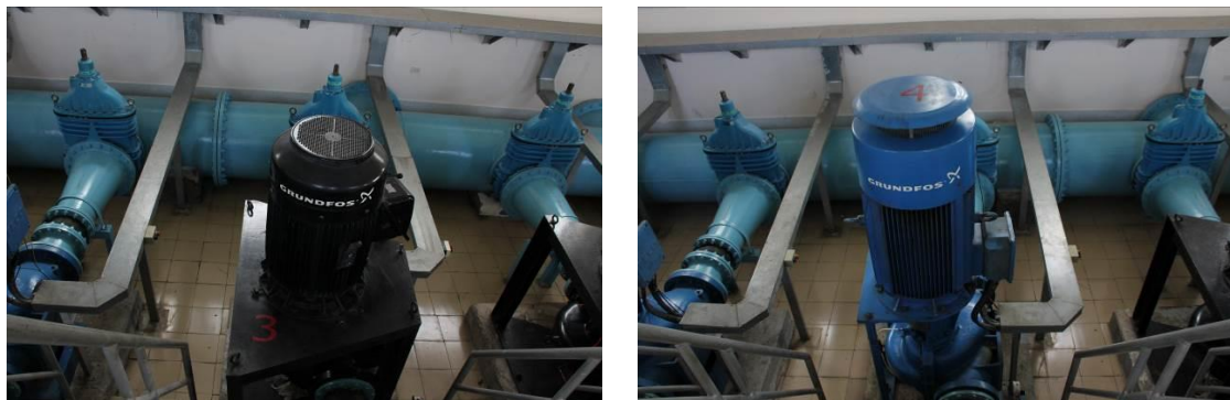
Figure 11 Distribution pump (black) and backwash pump (blue)
