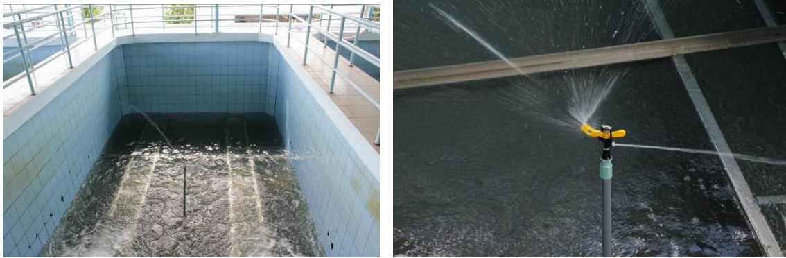
Figure 8 Another filtration tank with water spray to clean the wall
