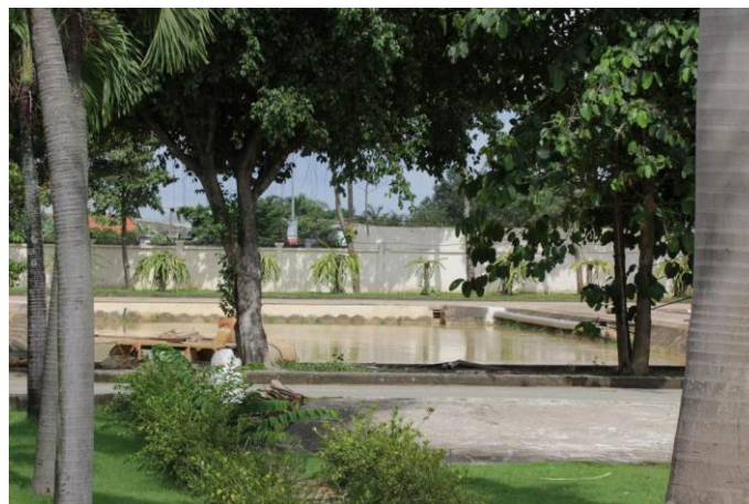
Figure 12 Sludge drying beds
