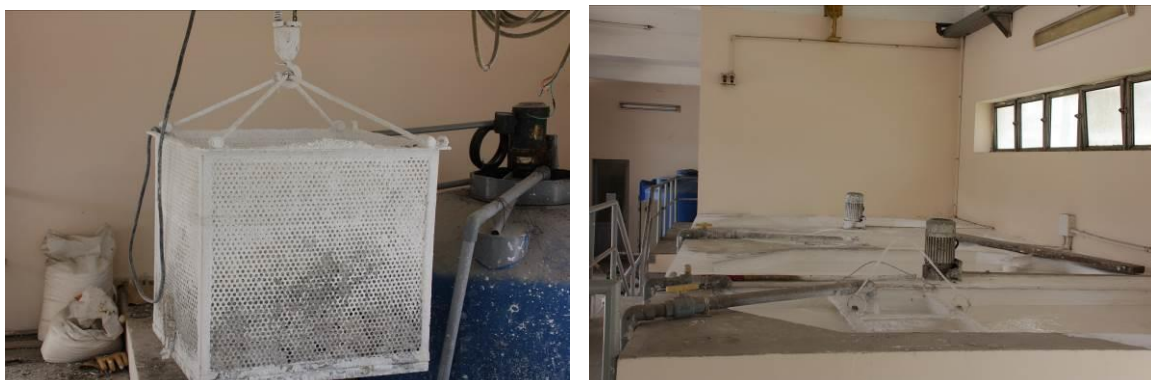
Figure 17 Lime dissolve tank
