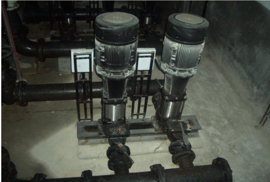
Figure 9: Medium pressure pumps
