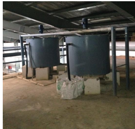
Figure 4: Alum dosing tank with mixer
