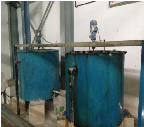
Figure 3: Chlorine dosing tank with mixer
