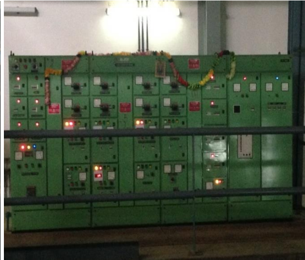
Figure 8 Control panel for backwashing
