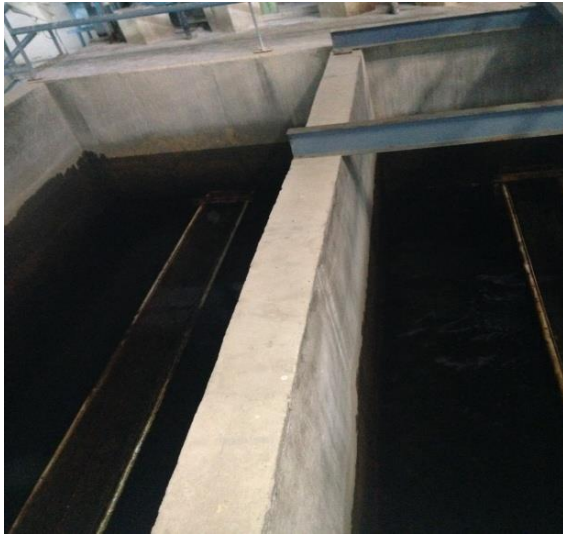
Figure 7 Rapid sand filter
