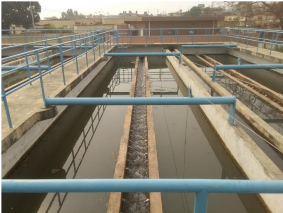
Figure 5: Sedimentation tanks (Rectangular shaped)
