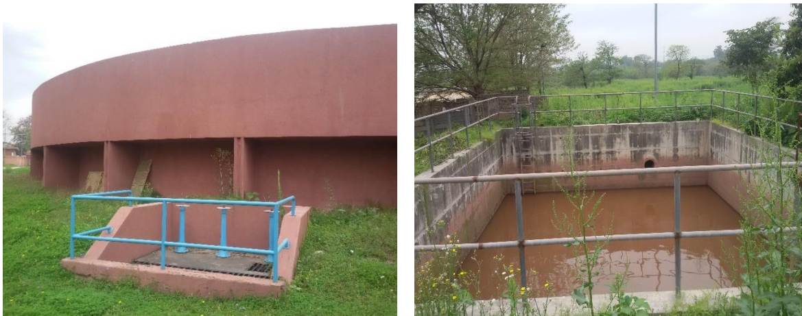
Figure 10: Sludge wasting Valves and collection basin
