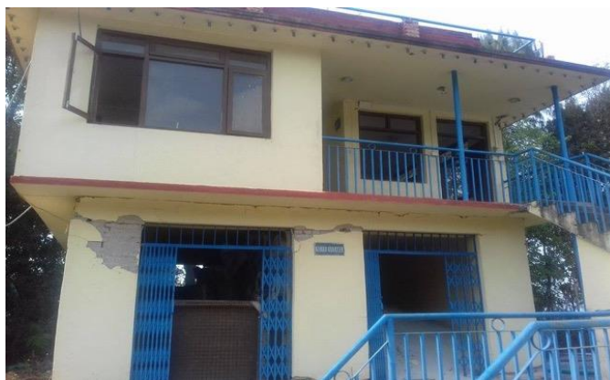
Figure 7: Water Supply Office damaged after earthquake
