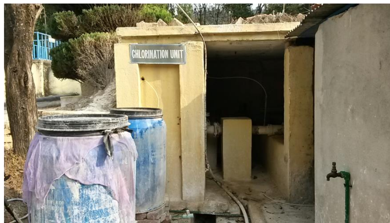
Figure 5: Chlorination unit and chemical storage room
