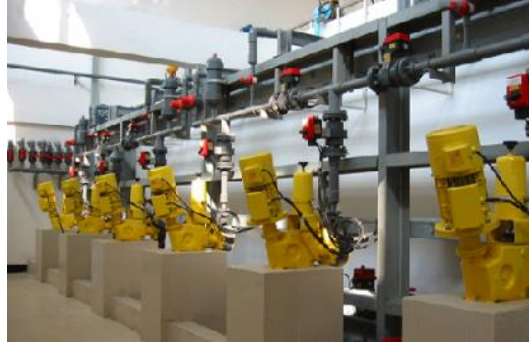
Figure 9 Coagulant aids dosing system
