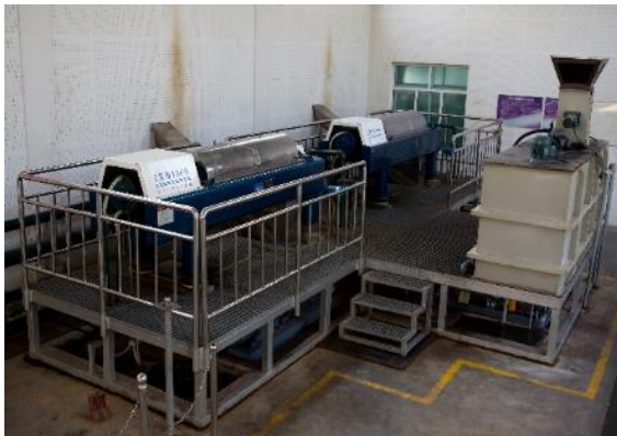
Figure 20 Centrifugal dewatering machine
