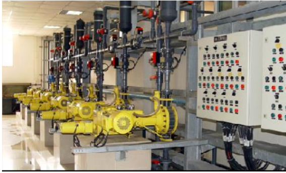
Figure 8 Coagulant dosing system
