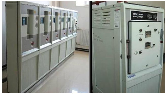
Figure 6 Chlorine dosing system
