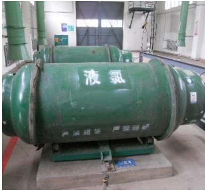
Figure 5 Liquid chlorine tank
