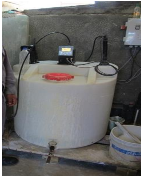
Figure 4 Chlorine dosing equipment
