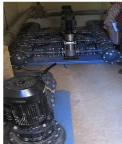
Figure 3 Pressure filter pumps
