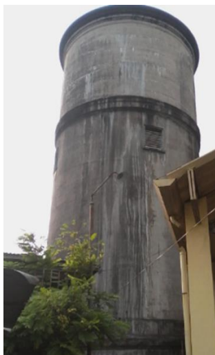
Figure 13 Water Reservoir at Burgos Pumping Station
