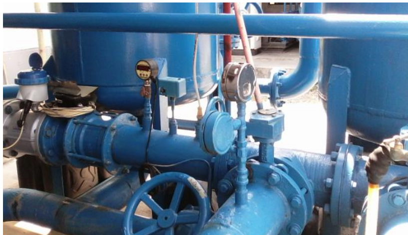
a) Injection Port for Disinfection at Fortuna Pumping Station
