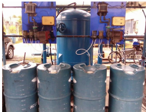
Figure 8 Chlorine dioxide Generation System
