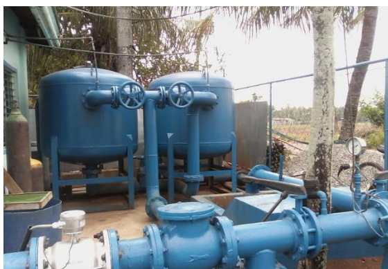
Figure 5 Bautista Pumping Station
