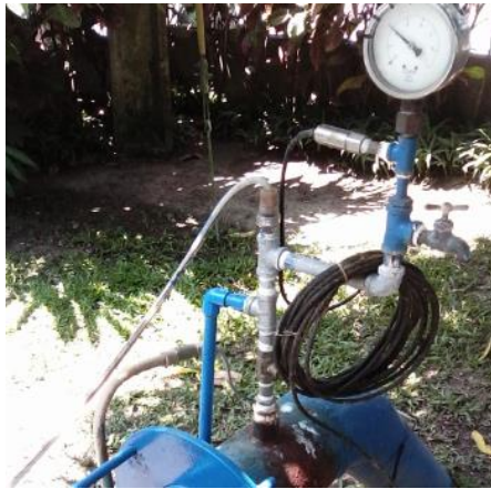
b) Injection Port for Disinfection at NJL Pumping Station
