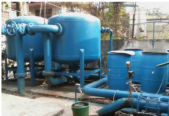
Figure 3 Burgos Pumping Station
