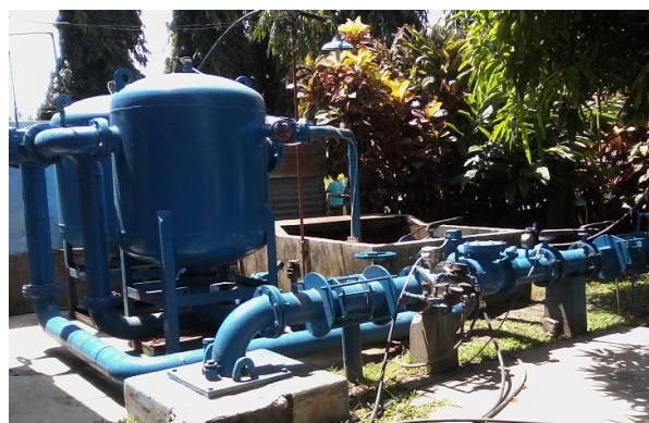
Figure 6 NJL Pumping Station
