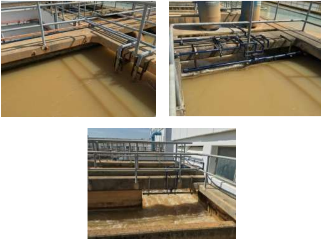
Figure 9: Pre Chlorine, Coagulant, and Flocculants Dosing Point
