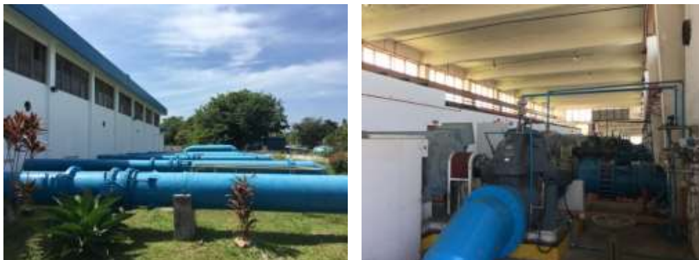
Figure 14: High lift pump for treated water distribution
