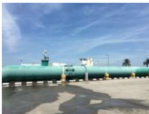
Figure 8: Low Lift Pump Pipe flow to Treatment Plant
