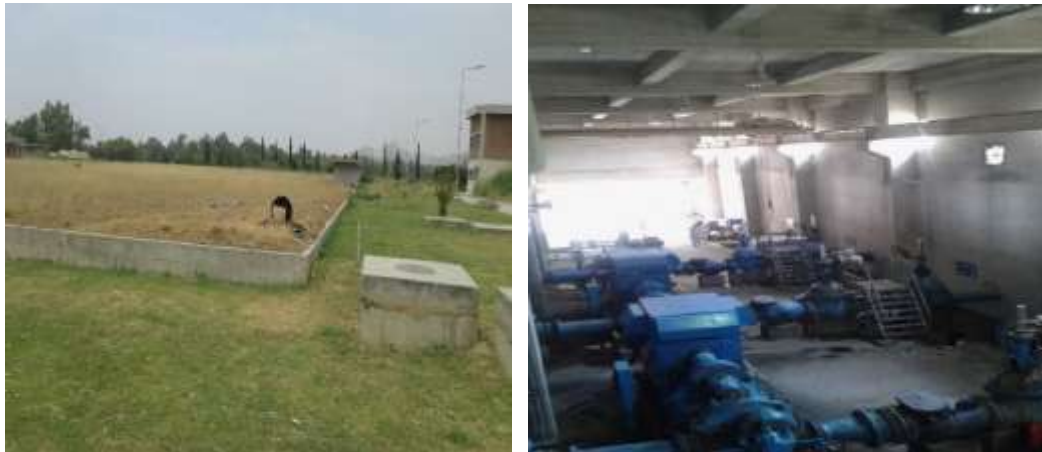
Figure 10: Clearwater storage tank and pumping station room
