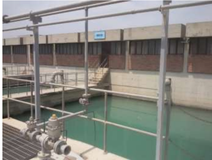
Figure 8: Rapid sand filter
