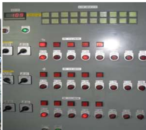
Figure 5 Control Panel for Backwashing
