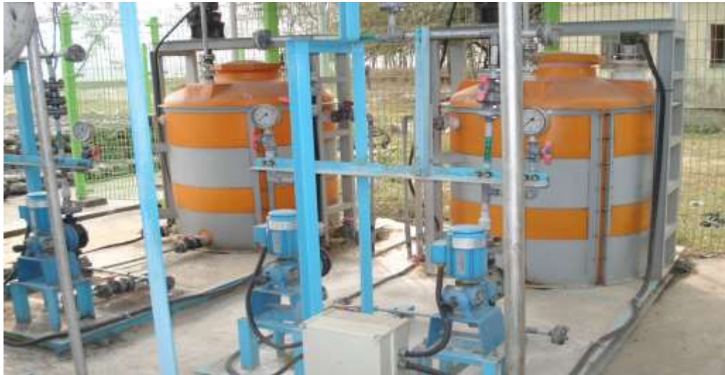
Figure 6 Chlorine dosing equipment
