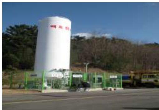
Figure 12 Facility of carbon dioxide injection in Bansong WTP
