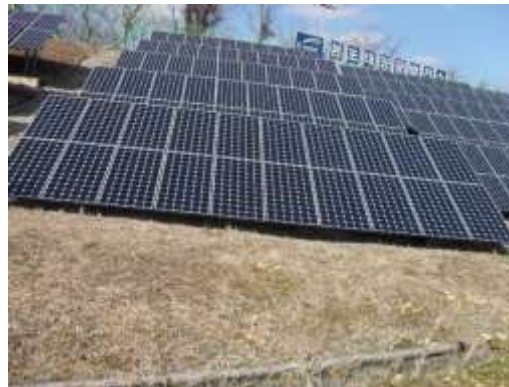
Figure 18 Solar panels installed at nearby water intake of Bansong WTP
