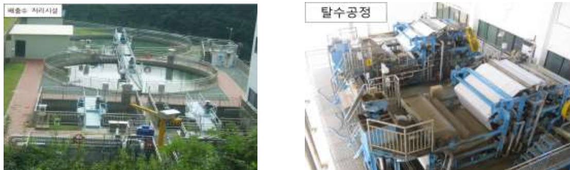
Figure 8 Gravity thickener (left) and dewatering machine (belt press)
