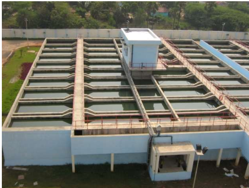
Figure 9. Clarified water collection channels of clarifier
