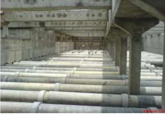
Figure 7. Distribution pipes of Pulsator clarifier
