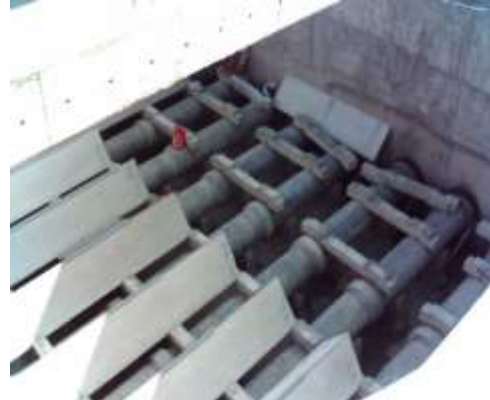
Figure 8. Distribution pipes with deflectors of Pulsator clarifier
