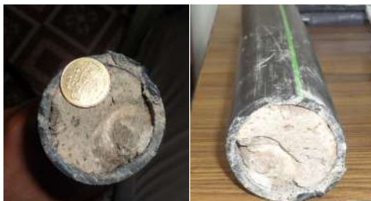
Figure 8: Calcification in drinking water distribution pipes (50 mm)
