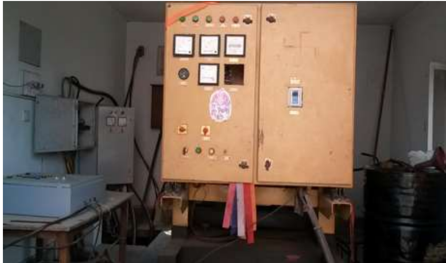
Figure 7: Generator (160 kVA) and electric switches for pumping stations
