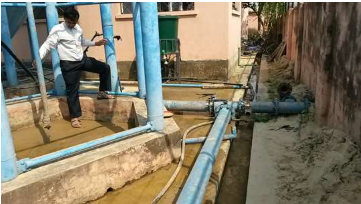
Figure 6: The silt deposit collected from the aeration tank
