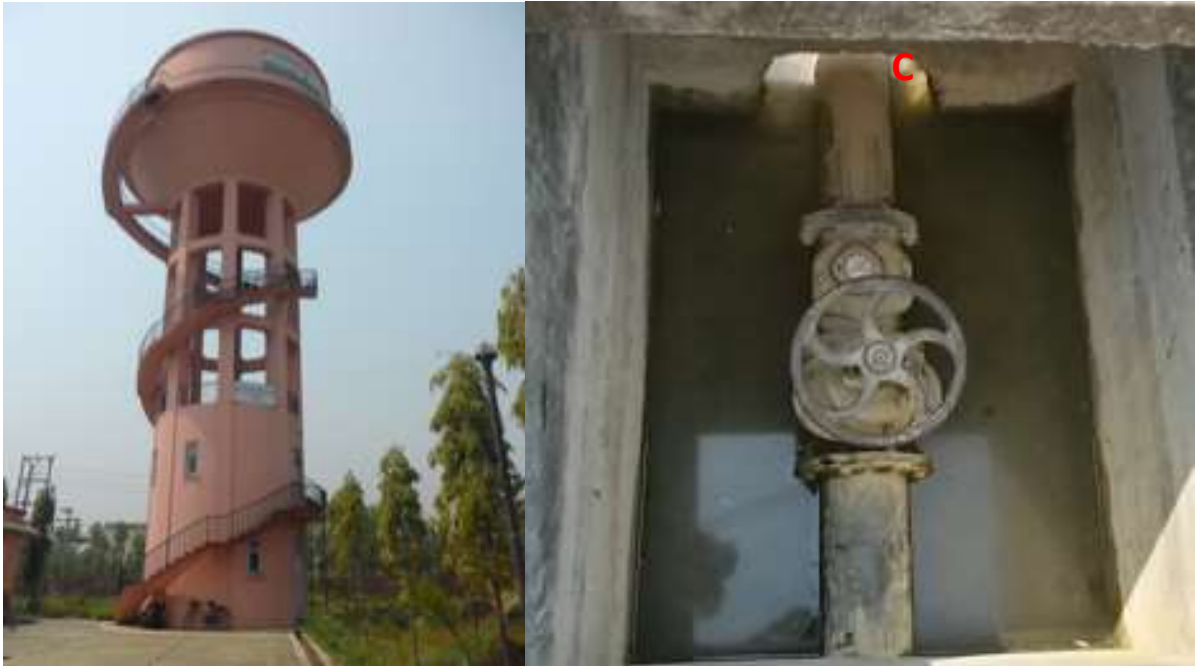
Figure 5: Over head tank of 450 m 3 (Left) and Gate valve for the water distribution network (Right)
