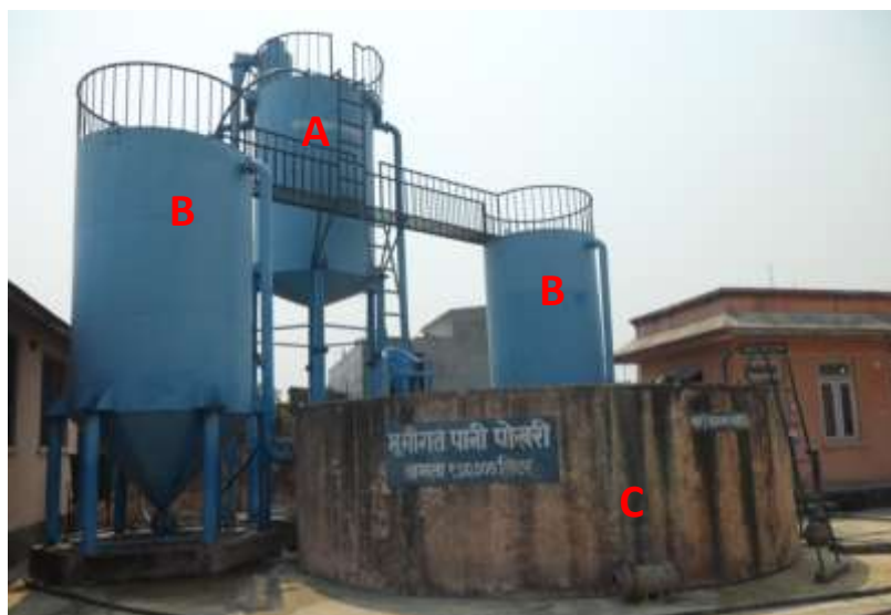
Figure 2: A – Perforated aerator (10 m 3 ); B – Sand filters and C – Underground reservoir (100 m 3 )
