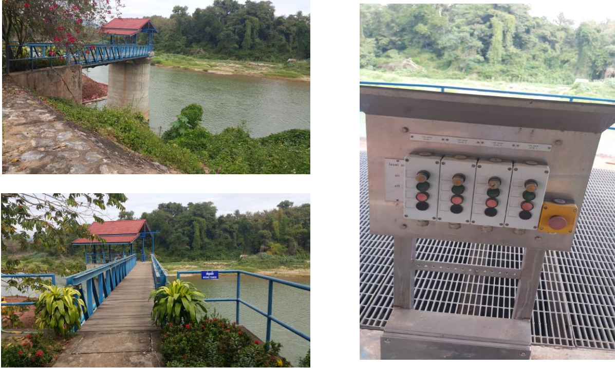
Figure 2 Khan river, pumping station (left), and bar screen (right)
