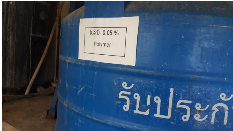
Figure 4 Storage Tank of Polymer
