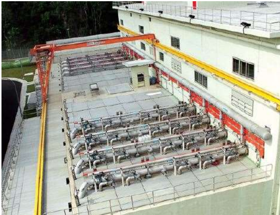
Figure 5 Siphoning to operate the UF process
