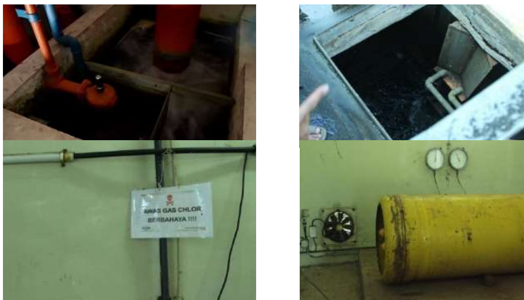
Figure 10 Chlor injection point and chlor storage room
