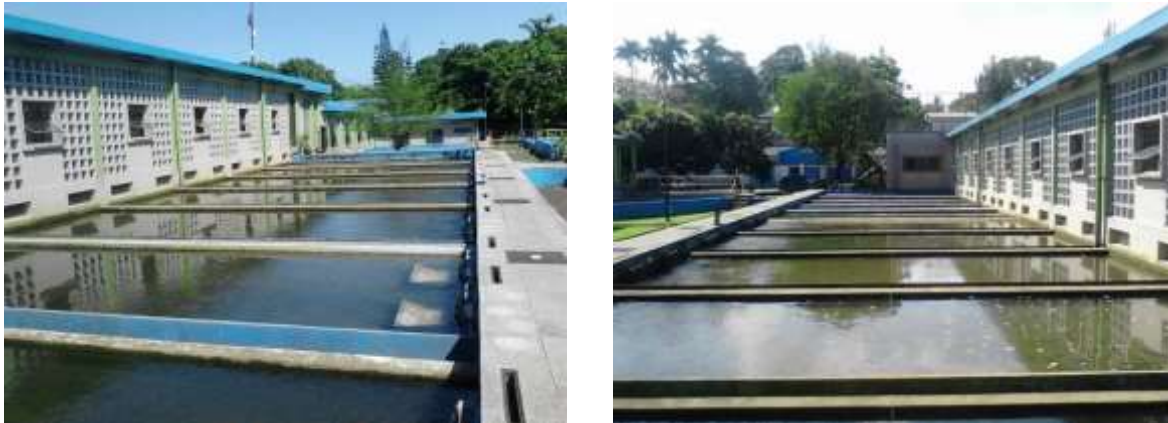
Figure 9 Rapid sand filter unit in Badak Singa WTP Source: Field visit, 1 st August 2016
