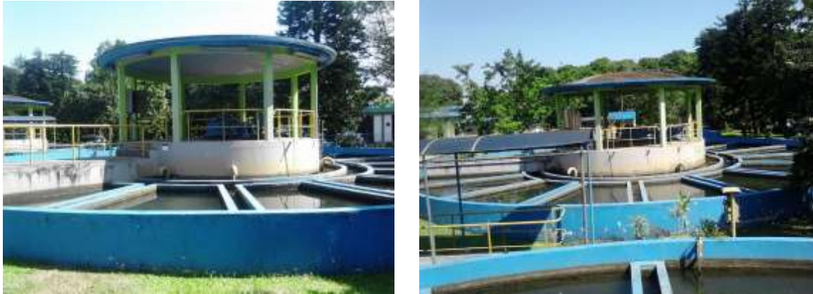
Figure 7 Accelators/clarifiers unit Source: Field visit, 1 st August 2016
