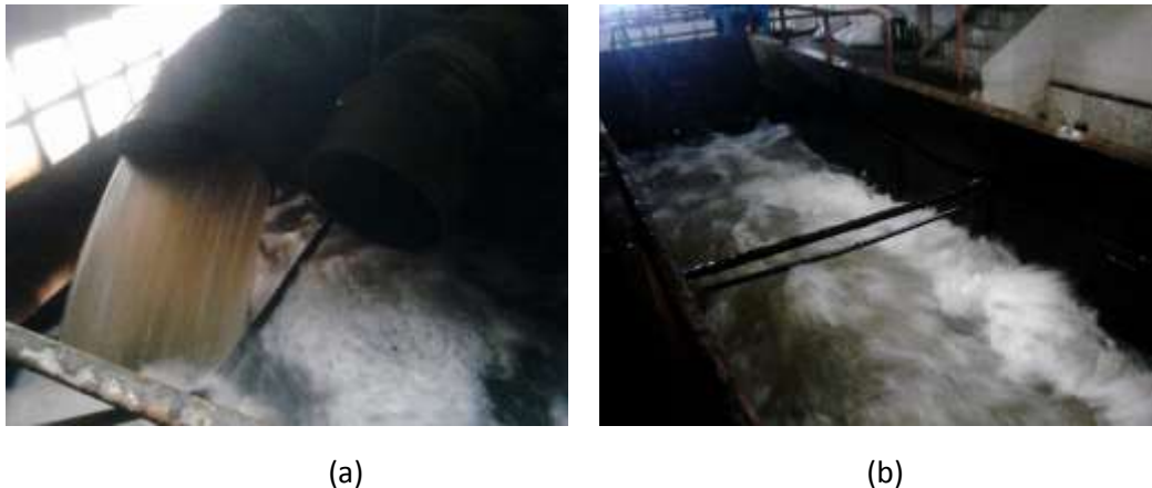
Figure 5 (a) Collecting chamber 1 receiving water from Cikapundung river, and (b) collection chamber 2 receiving water from Cisangkuy river with bar screen Source: field visit, 1 st August 2016
