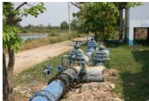
Figure 4 Static mixing of alum, lime, and pre-chlorine
