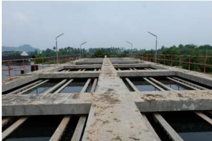
Figure 7 WTP sedimentation basins
