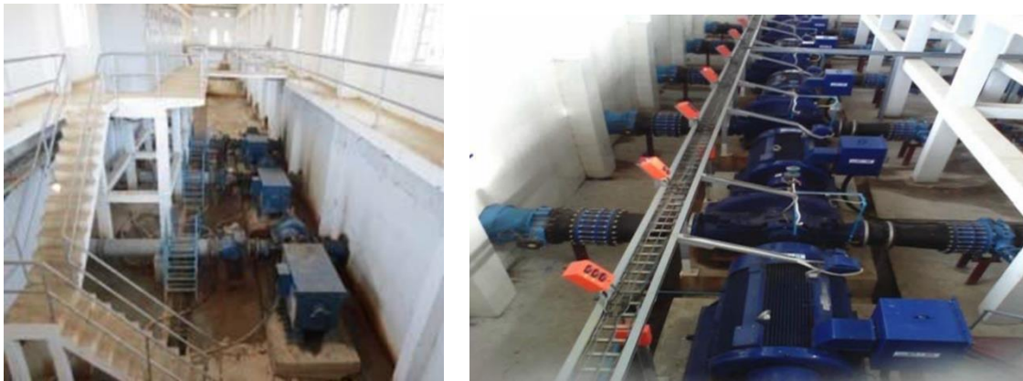
Figure 16: Pumping stations in Nyaungnapin WTP
