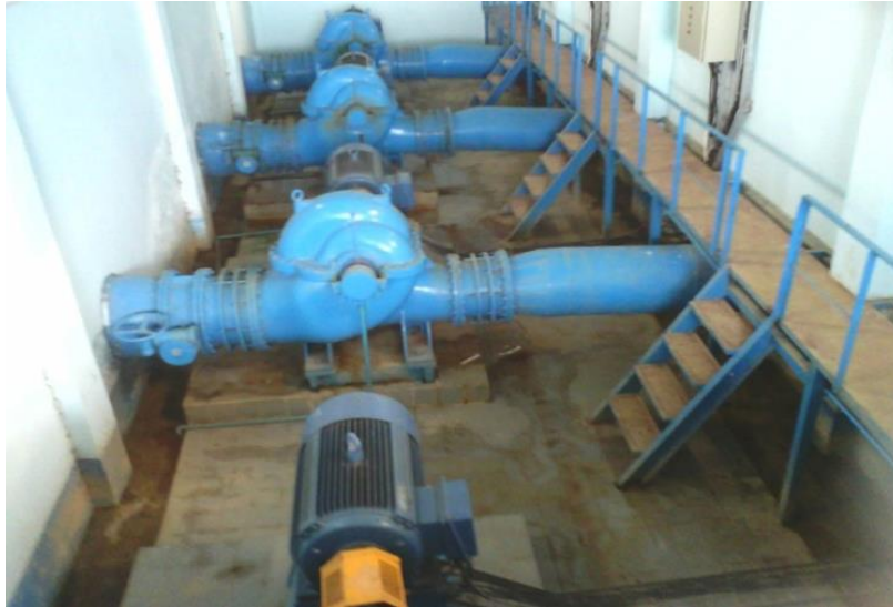
Figure 6: Pumps to lift water from pre-sedimentation tank to water tower
