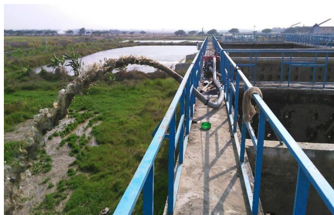
Figure 17: Discharging sludge from the sedimentation tanks
