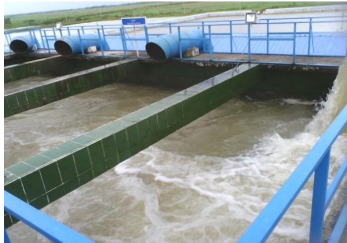
Figure 7: Incoming water into the water tower
