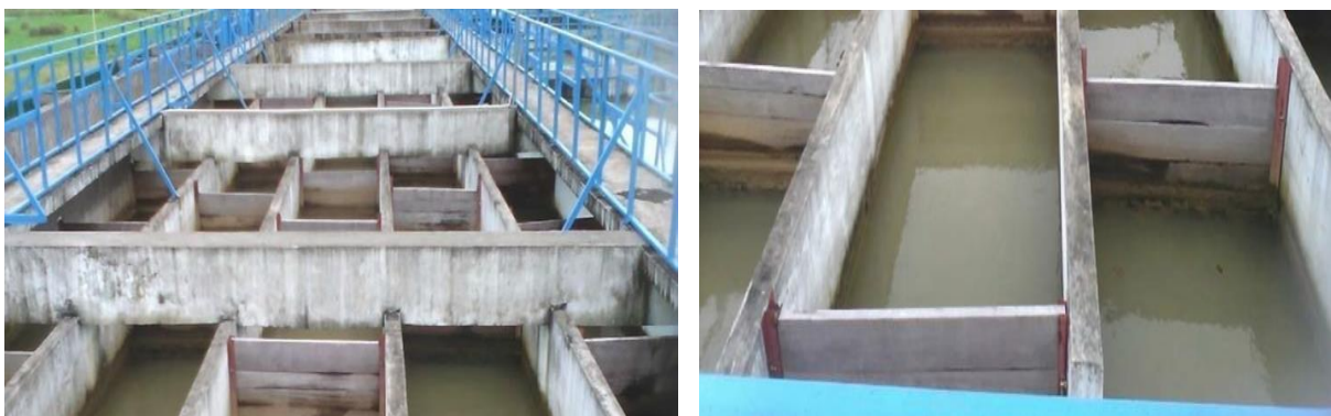
Figure 9: Flocculation unit (vertical baffled tanks)
