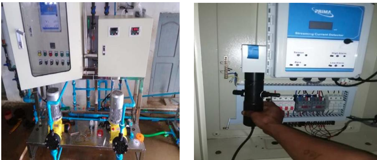
Figure 11: Chemical injection equipment
