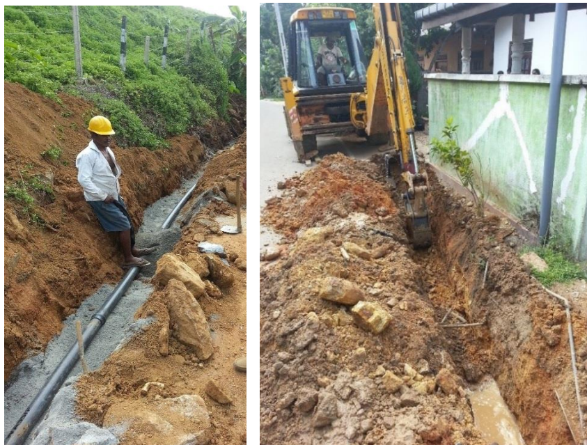
Figure 3: Laying of pipelines under Garagoda Rural Water Supply Scheme as a part of WaSSIP
