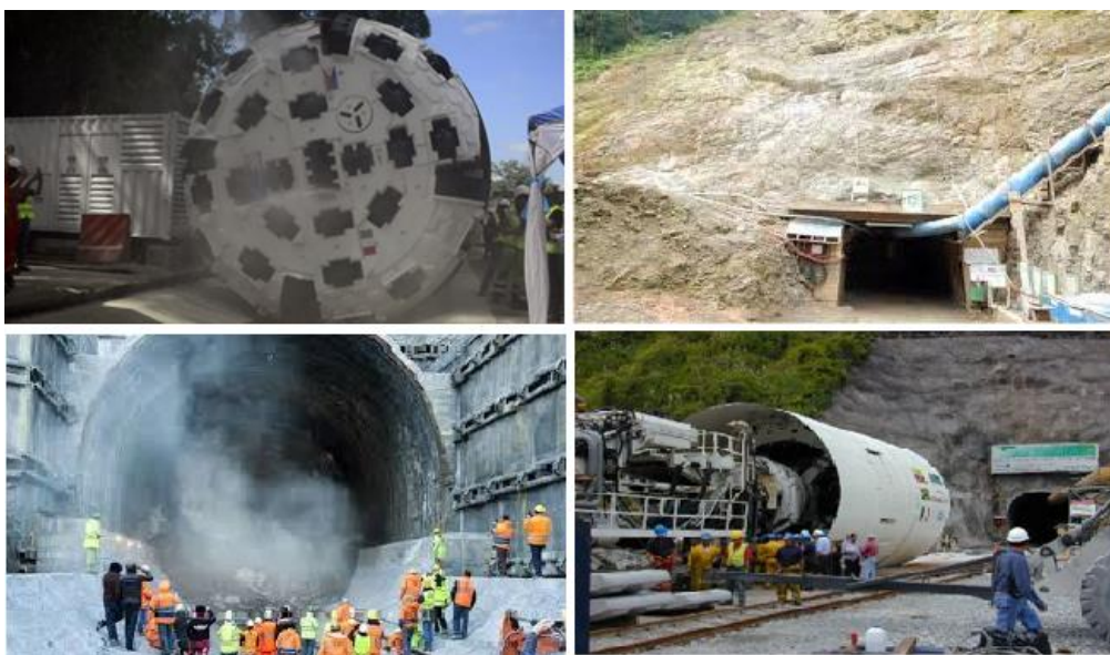
Figure 4 New tunnel construction using modern bored tunnel methods on the AWTIP (Source: mwss.gov.ph )
