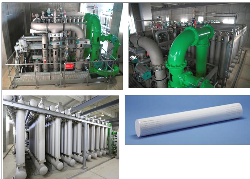
Figure 4 | Membrane filtration facility at Kawai
